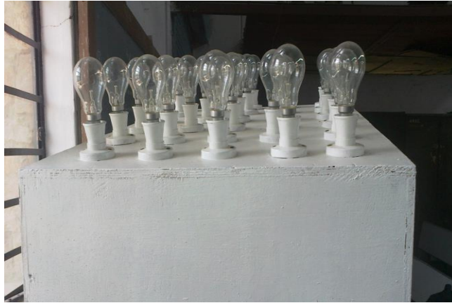
Figure 4: Connection of bulbs on load bank
